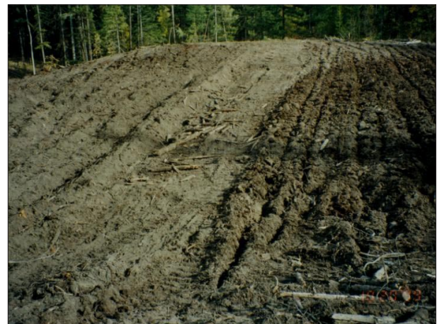
FIGURE 1. Landing rehabilitation. Burn-pile debris and recovered topsoil incorporated via ripping (left) or landing simply ripped (right).
