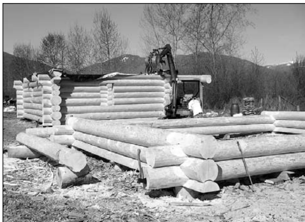
FIGURE 2. Log house components are manufactured on site at the Creston Valley log sort yard.
