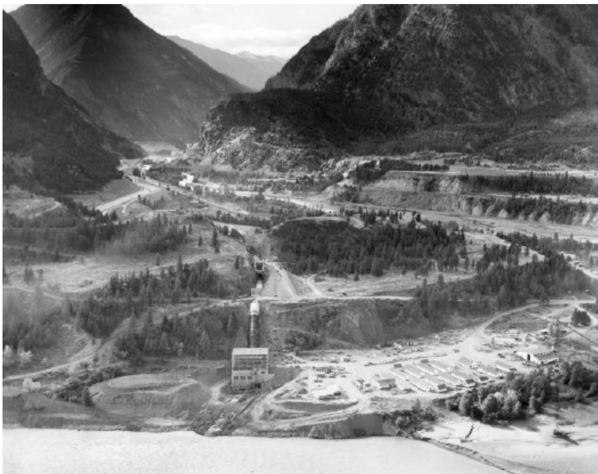
FIGURE 1. Disturbance on the grand scale: construction of the Seton Dam and Powerhouse in the 1950s. The Fraser River is in the foreground.
